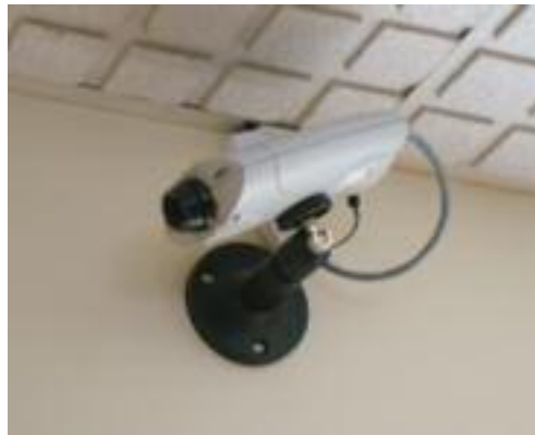
FIGURE 48. Webcam positioned above armoury entry doors
