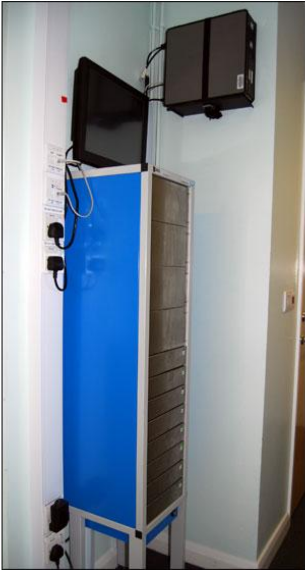
The cabinets have drawers, each of which stores a specific Taser and its cartridges. The drawers remain locked until being authorized to open by an officer presenting an RFID badge to a reader (on right).
